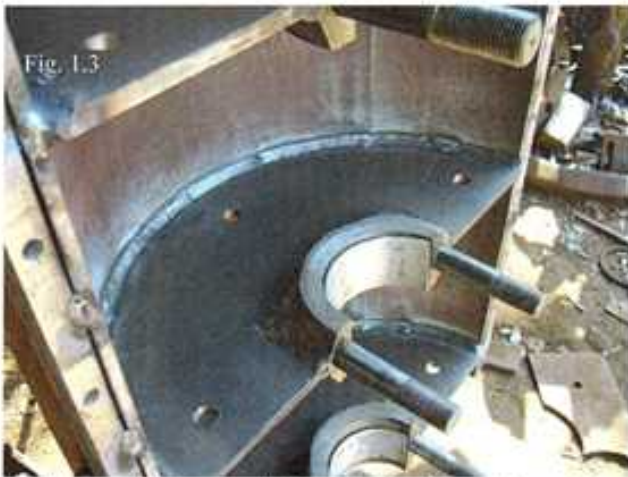
Fig. 1.3 Close-up of the weld holding the webs and main bearing housings in place.
