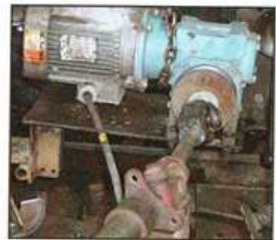
(Above) Nev's improvised motor and reduction gearbox used to drive the line boring apparatus via two universals.
