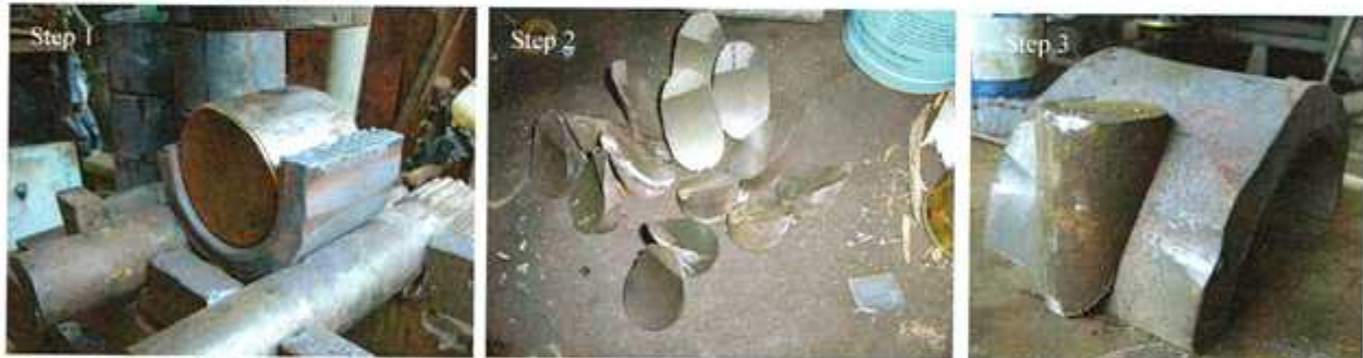
Steps involved in forming the main bearing housings. 1. Shaping the 3"x1" flat steel by pressing them to form semi circles. 2. Bolting flanges were fabricated. 3. They were then welded on to the housing bodies. Holes were later bored through the flanges so they could be bolted together in pairs to form the main bearing housings.
