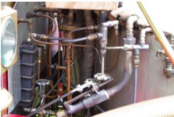
A view of the back of the boiler.
